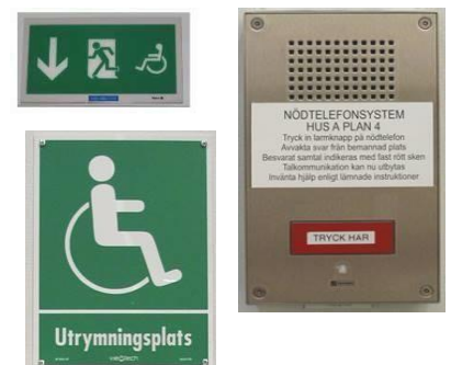
Fig 6. Temporary evacuation station
